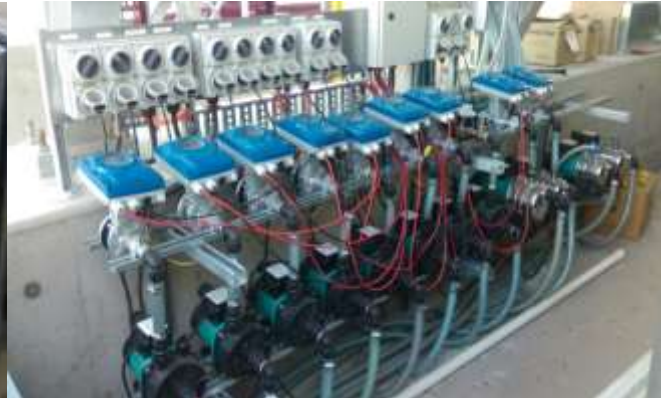
KMS502-25F 25mm flowmeters install
