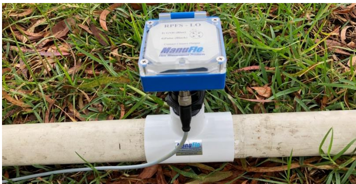
RPFS-LOD installed on a 50mm PVC pressure pipe line using PVC50 adaptors.
